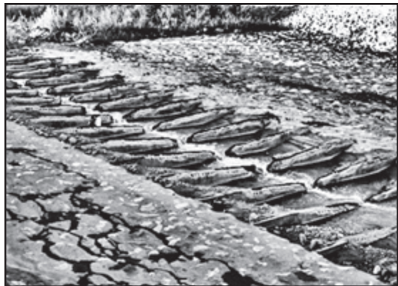
The failed fishladder on Santa Paula Creek. The Army Corps proposes to build a similar fishladder right beside it.
