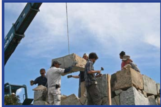
As the masons finish the west rim of the west rampart, the view up the hill from the cross now shows two finished rampart fronts. Note the graceful way the ramparts narrow to the top, and how beautifully the rock jigsaw puzzle fits together. The rows of holes on some of the rock edges in the right rampart are visible signs of a traditional Japanese rock-splitting technique.
